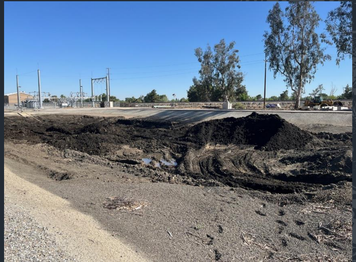
Shallow Groundwater Encountered
